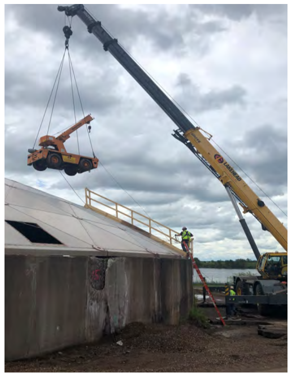
A crane lowers machinery into a clarifier, the St. Louis River estuary is pictured in the background.
